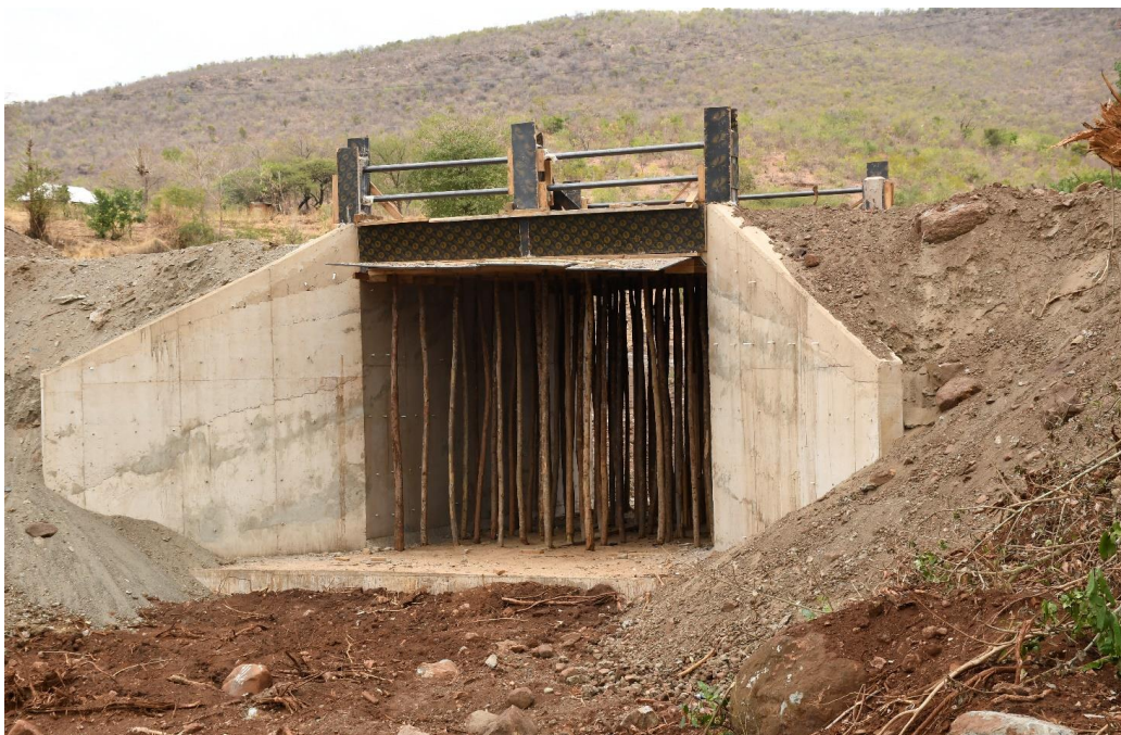
Box culvert lililopo barabara ya Babati – Mutuka
